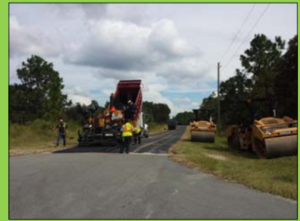
W. Pinegrove Drive at W. Swanson Drive; placement of first course of asphalt
