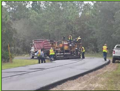
N. Parkview Drive at N. Shafton Terrace; placement of final surface course
